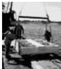
Anode beds were lowered to the sea floor to counteract the effect of the stray currents.
