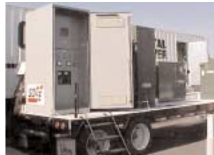
EPRI's DR field evaluation project systematically evaluates the performance, siting, and gas supply considerations of diverse new power generation and storage technologies.
