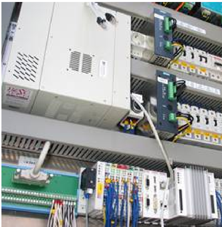
Figure 15: Transformer monitoring and merging unit IEDs
